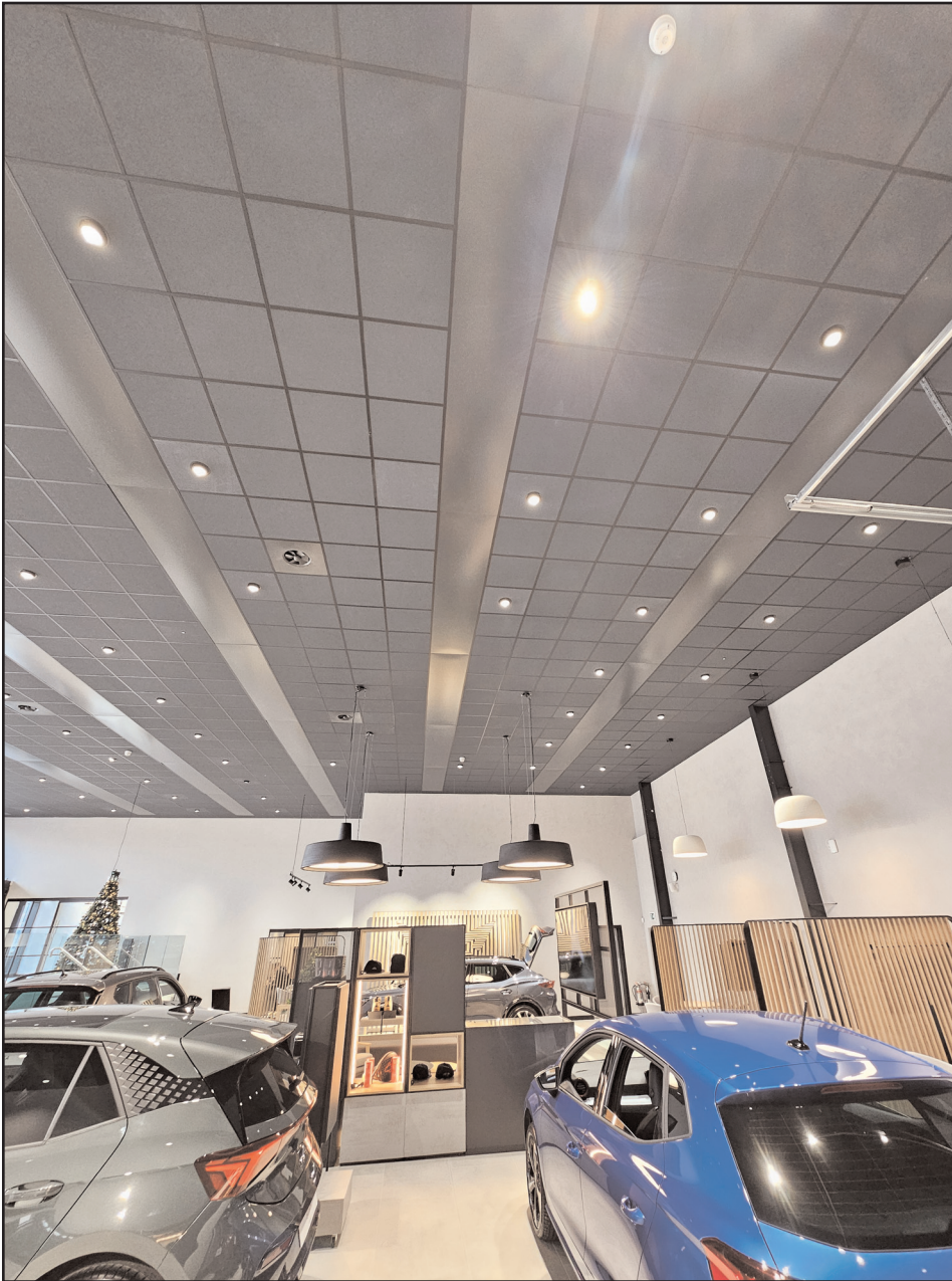
Colman's LQS tile replacement diffuser installed at JCMG Cupra, Aberdeen.
